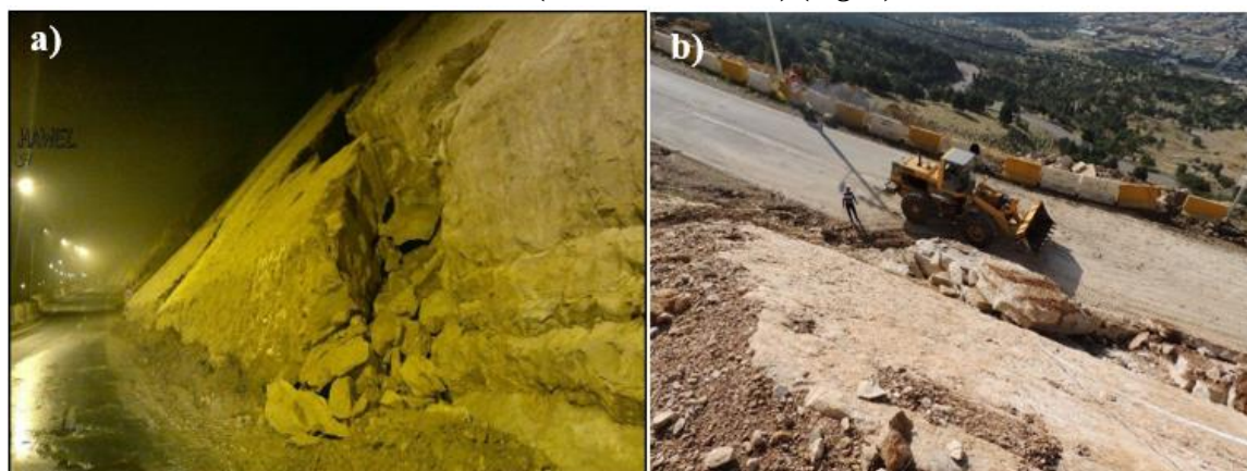
Fig. 1. Slope failures at Haibat Sultan Road: a) on 14.12.2013, b) on 8.5. 2016
